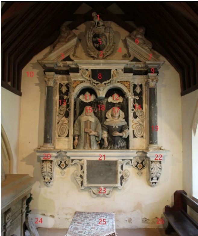
Figure 17 Surface Moisture readings on North Chapel Wall & Monument
