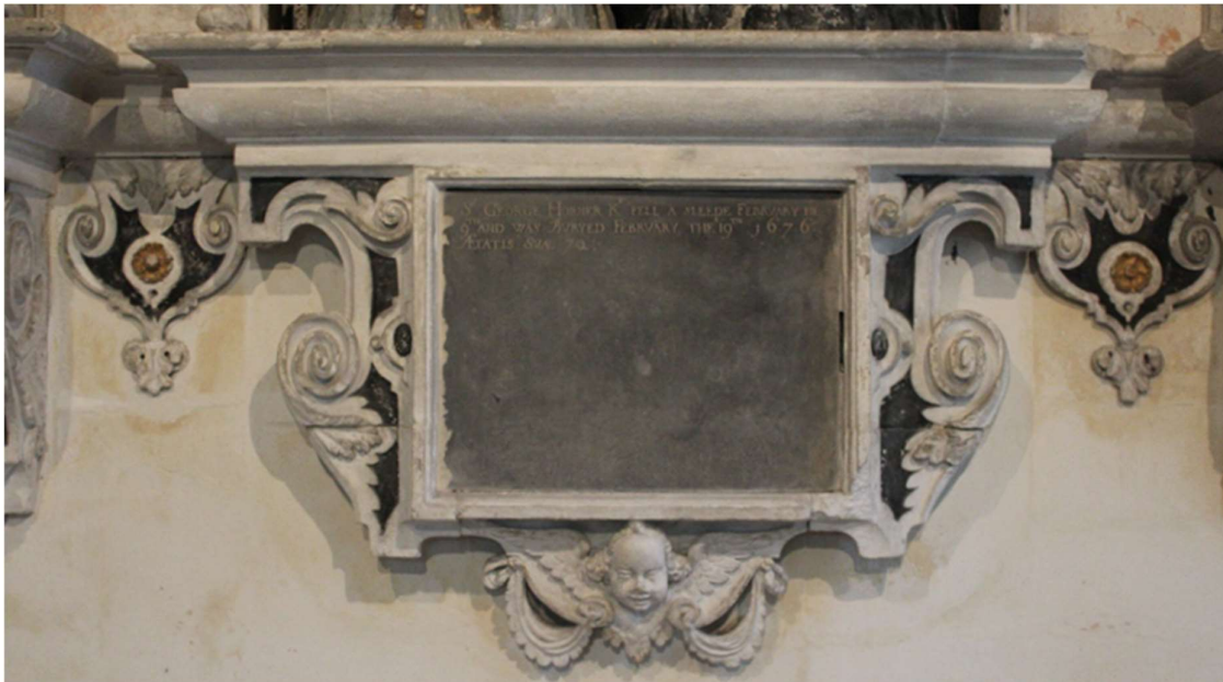
Figure 58 Monument with the missing grape and leaf embellishments
