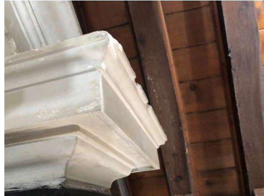
Figure 79 Sinister cornice (before repair)
