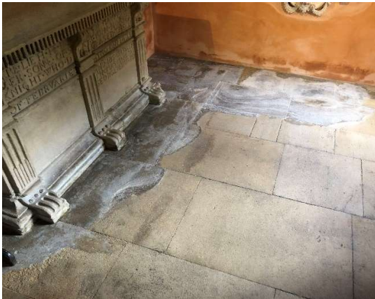
Figure 83 Salt formation on the stone floor in the north-west corner; September 2022
