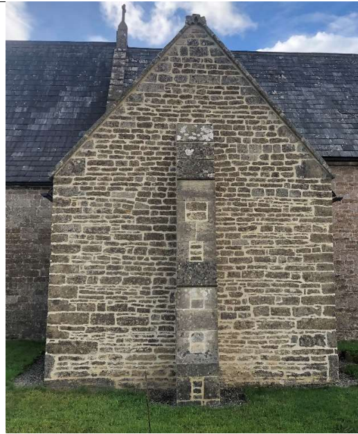
Figure 88 The current view of north wall of chapel, new pointing revealing historical interventions
