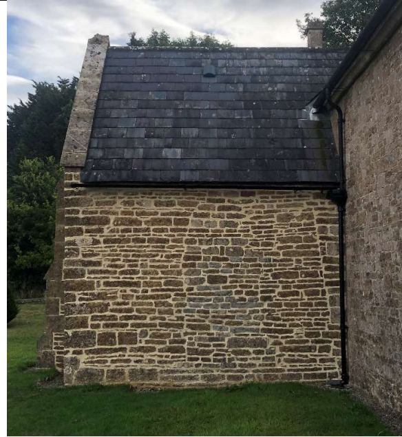
Figure 86 The current view of west wall of chapel, new pointing revealing historical interventions
