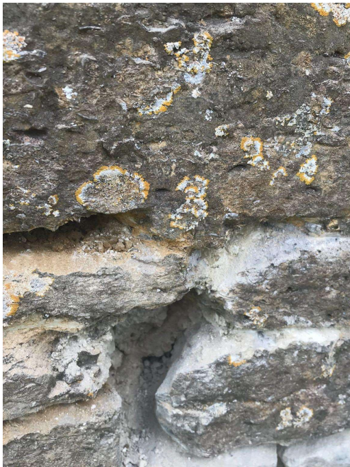
Figure 2 Image to show hard cementitious mortar to the right and softer lime mortar to the left.
