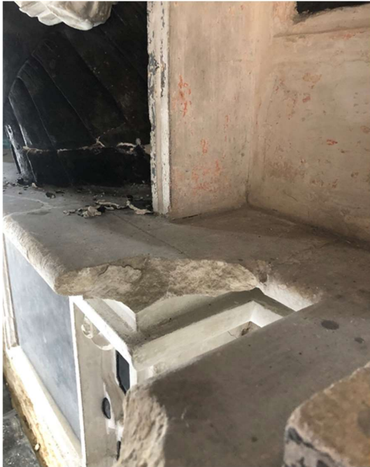
Figure 45 Missing sinister section of main mantle
