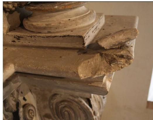
Figure 48 Missing section before repair to the far sinister mantle
