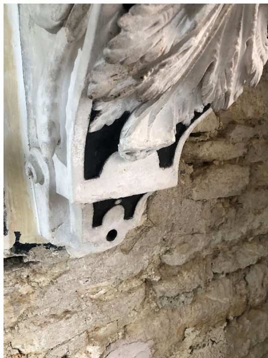
Figure 51 Missing leaf on sinister corbel
